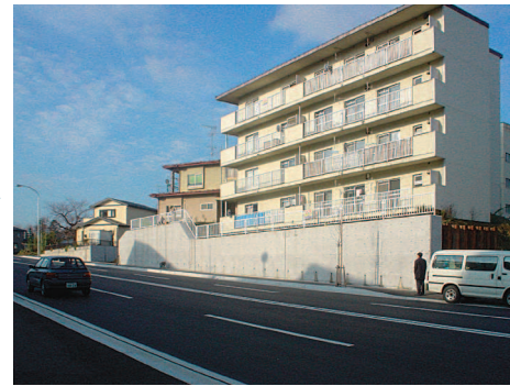
Steel sheet pile wall is covered by concrete panels to conform to the neighboring view.
